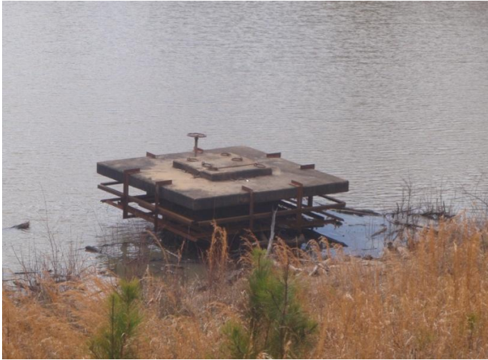
Figure A-5 The tunnel entrance from the on the north side of the tunnel
