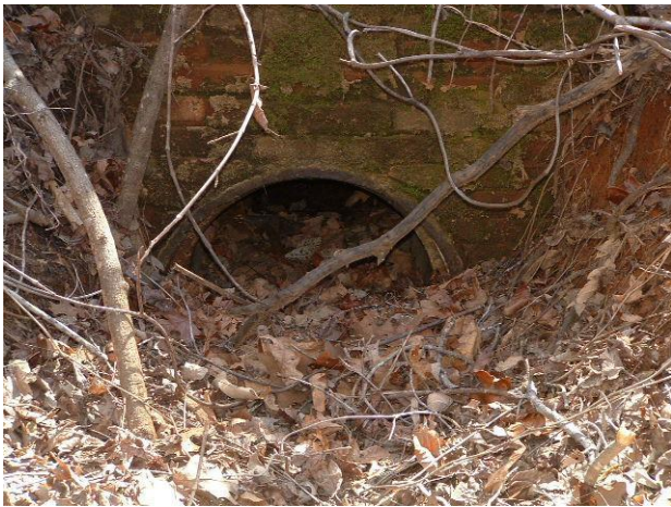
Figure A-12, this is the north side of the tunnel 5, the culvert is partially filled
