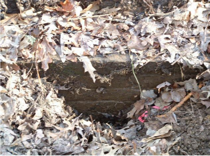
Figure A-17 This is the north side of the tunnel, it is partially filled
