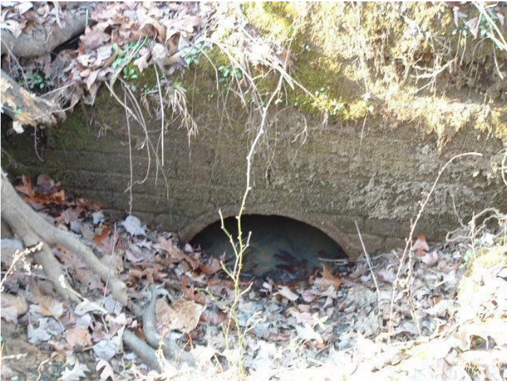
Figure A-18 This is the south side of the tunnel, there is a mixture of water, leaves and tree branches in the tunnel.
