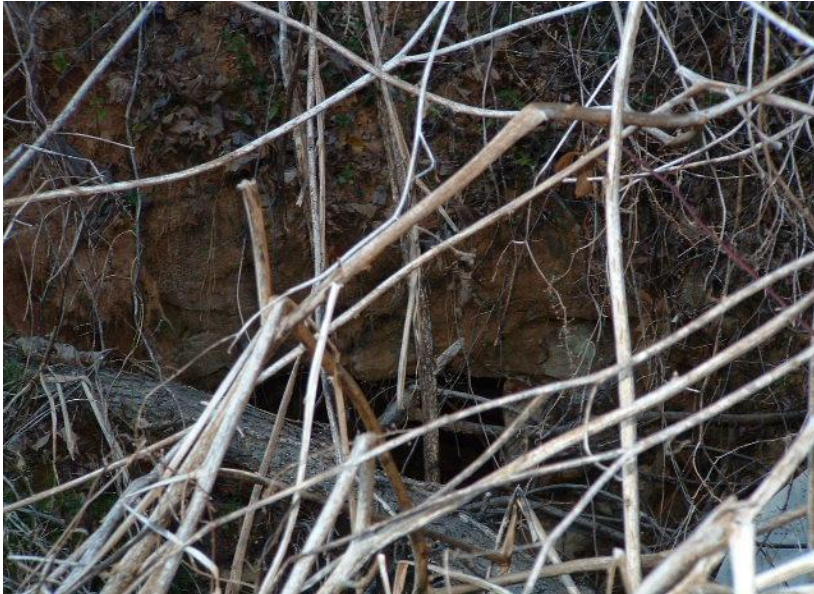
Figure A-14 The south side of tunnel 6, the tunnel was completely covered , but is not filled
