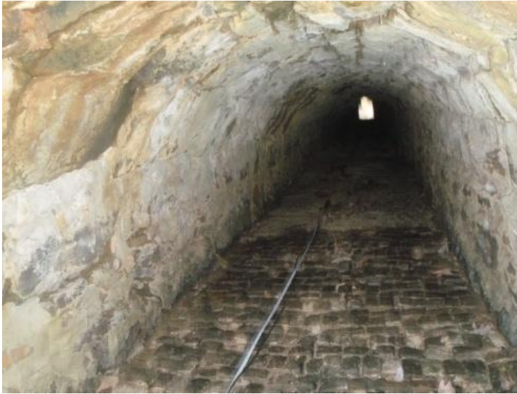
Figure A-1 This is the a picture of inside f tunnel 1. On the ground is a measuring tape used to put the 3-C geophones inside the tunnel during acquisition
