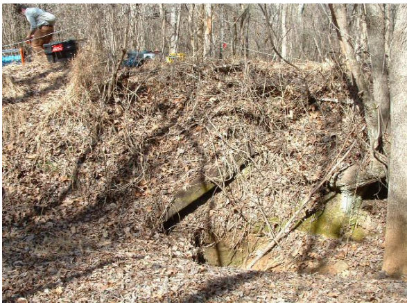
Figure A-13, this is the south side of tunnel 5. The tunnel is partially filled.
