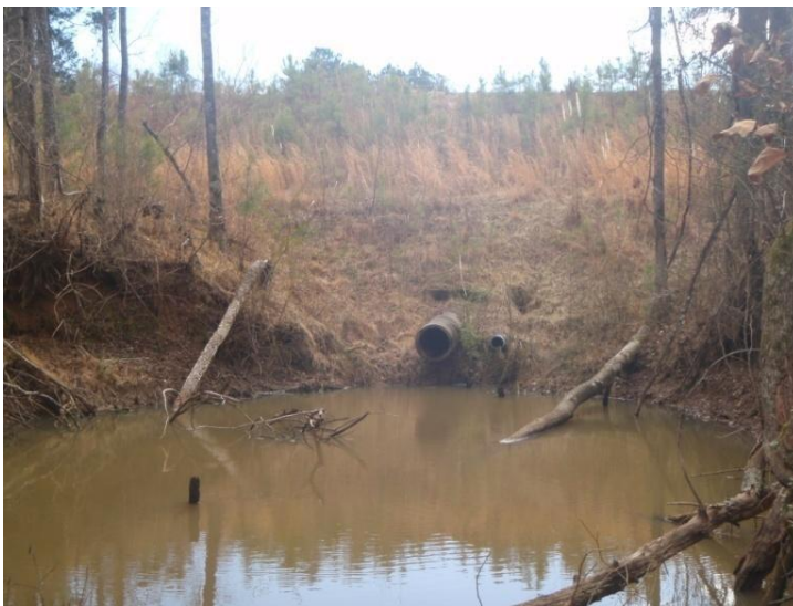
Figure A-6 the tunnel on the south side with the towards the drainage zone.
