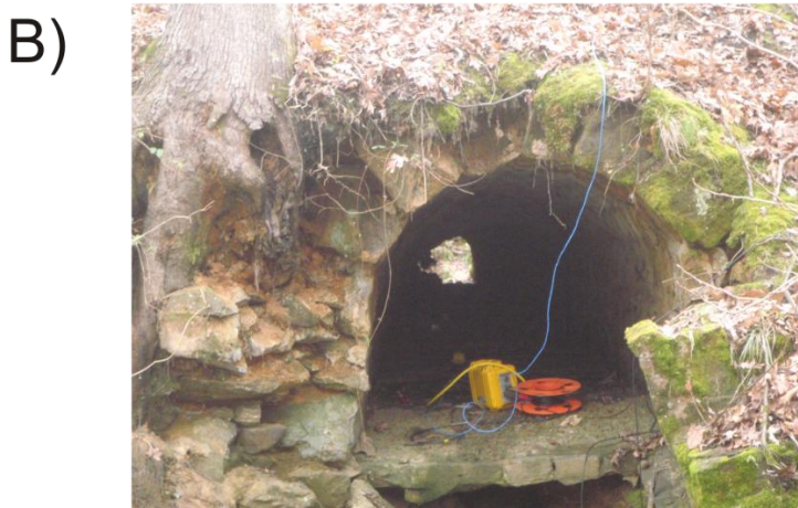
Figure 3-2 A) this is the subsurface view for the general railway site. The tunnel casing changes on a site per site bases. B) This is a picture of the tunnel 1 in Oxford, MS can see a sandstone blocks as casing along with a geode spread through the tunnel.
