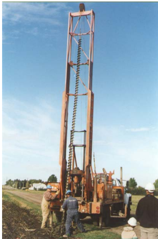
Figure 4.2: An auger drill rig was used to obtain soil cores at the University of Alberta Edmonton Research Station (drilling done by Mobil Augers).
