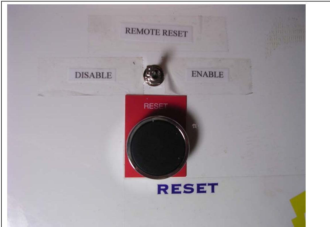
Figure 1: The RESET button on the GridTek10 is a NC switch. Pushing the button causes an open circuit condition that causes the reset. The toggle switch (SPST) above was added to enable or disable the REMOTE RESET. See details below.
